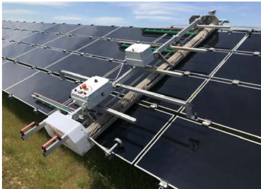
Figure 1: Cleaning Robot in operation
